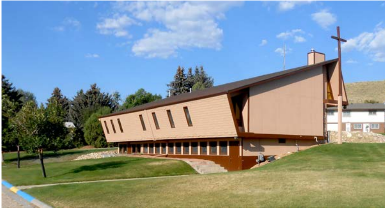
New roof and new paint. The walk-out basement of the parsonage is shown in the right-hand side of this photo
